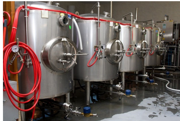
Beverage processing plant production line
