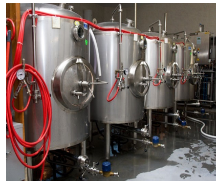
Beverage processing plant production line
