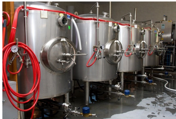
Beverage processing plant production line
